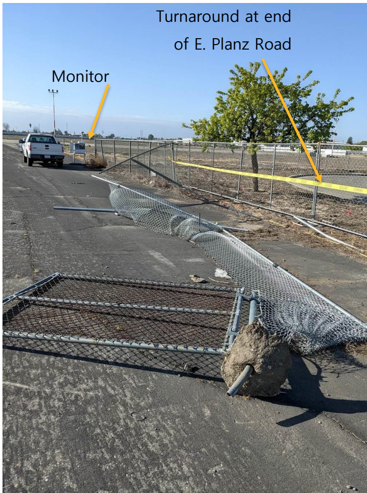
Figure 3. Fencing near Planz Monitor Damaged by Accident
