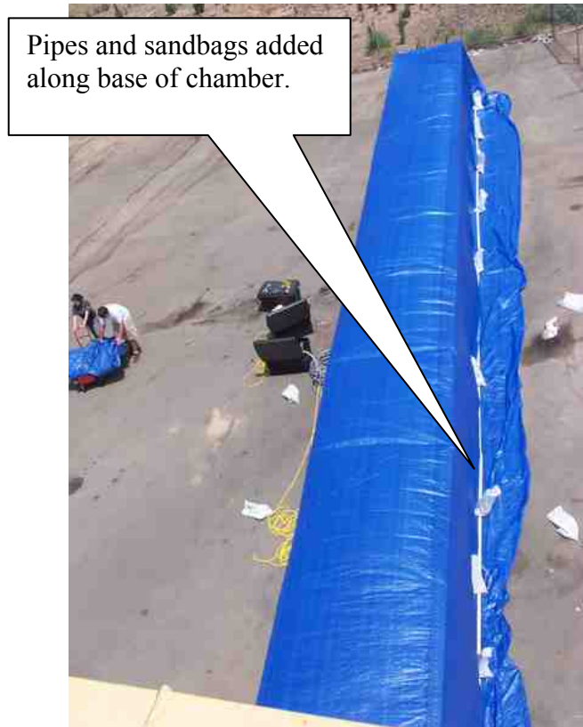
Figure 13. Addition of pipe and sandbags along base of chamber to eliminate leaks.
